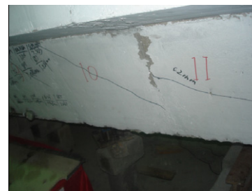
(c) diagonal cracks
