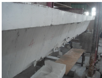
(a) no cracks under a small load
