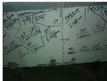
(e) crack propagation
