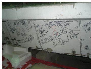
(d) further opening of joints crushing
